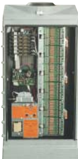
Intelligent, attractive Field Controllers feature clean, modular layouts for easy expansion and diagnostics
